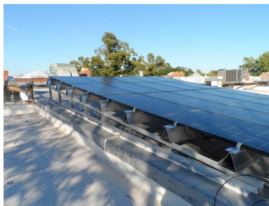
Solar Panels on DC townhouse
